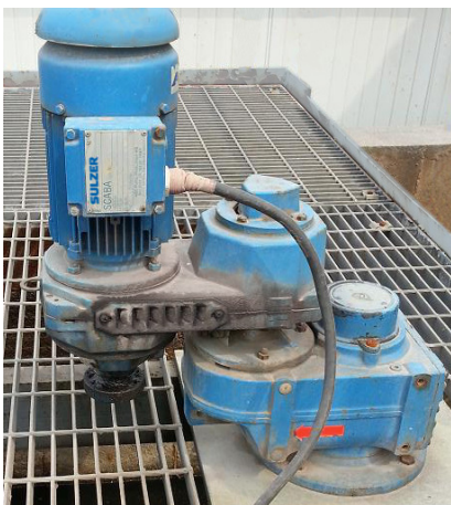
A top-mounted Scaba agitator installed at the Asia Symbol (Shandong) Pulp & Paper Co., Ltd in China contributes to reliable operation in the wastewater treatment process.
