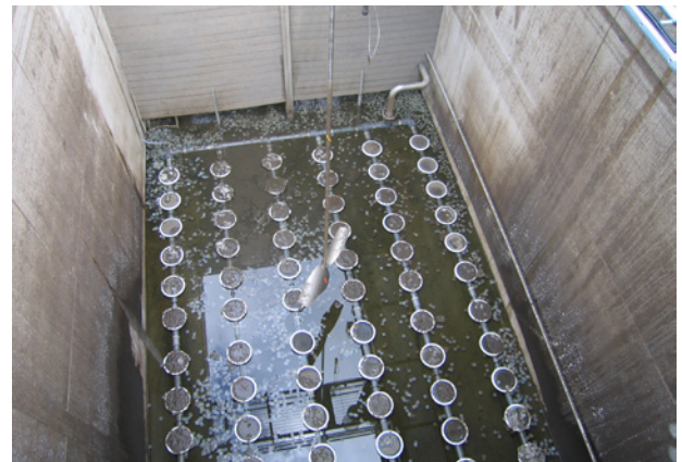
Denitrification can be an intermittent aeration process with anoxic and aerobic phases created alternately.
