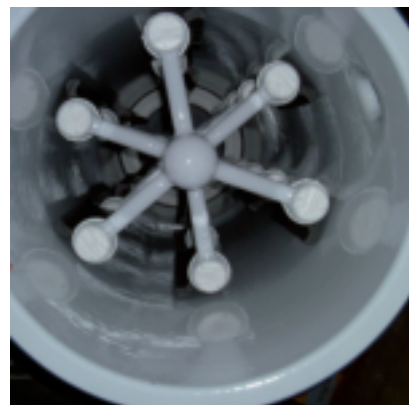
Inside of a glass-lined evaporator
