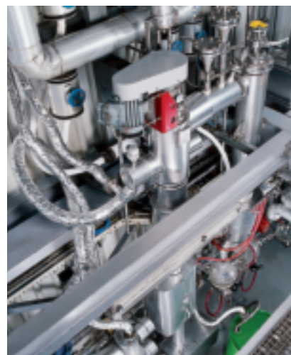
Pilot unit of a thin film evaporator in our test center
