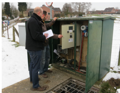
The controls of a pumping station at Honthem.
