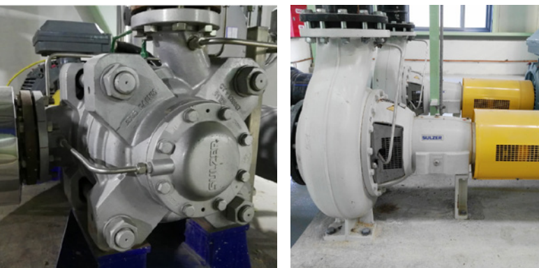
Auxiliary pumps completed the range of assets that Sulzer installed
