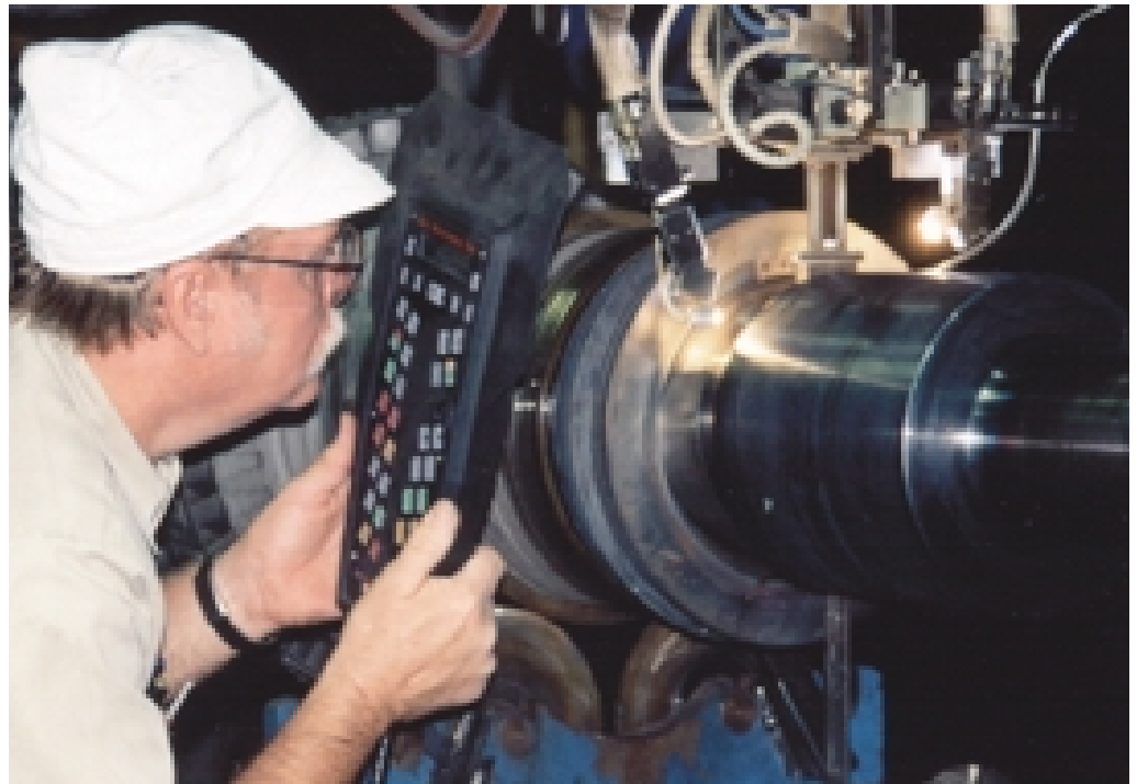
5 ■ A weld repair technician with remote pendant is finalizing a 30-MW steam turbine rotor shaft end.
