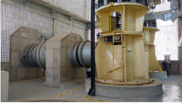
The completed pumps were installed and commissioned by Sulzer's field teams
