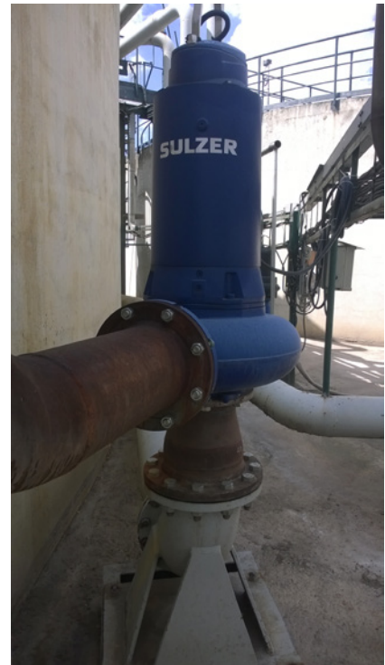
A dry-installed XFP 201G-CB2 PE110/6 pump for sludge recirculation
