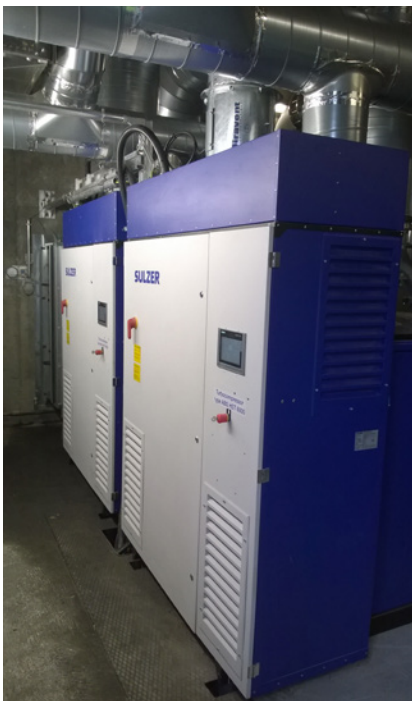
Sulzer HST 6000 turbocompressors
