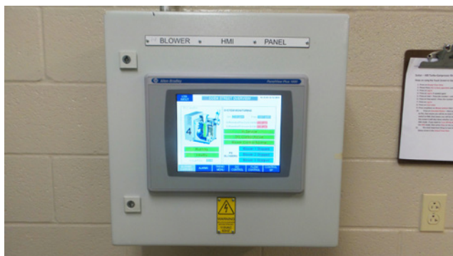
HMI screen moved inside building
