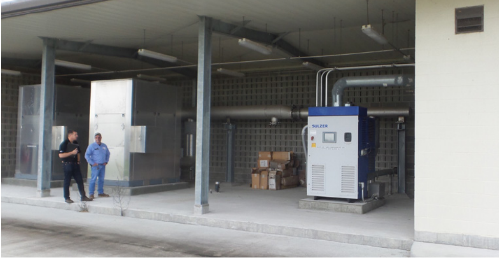
Sulzer HST 2500 alongside existing centrifugal blowers
