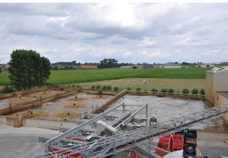
Biological basins where OKIs replace surface aerators.
