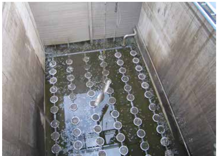
Denitrification can be an intermittent aeration process with anoxic and aerobic phases created alternately.
