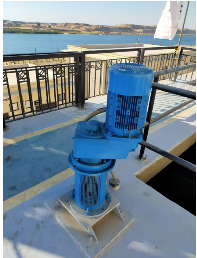
Sulzer specified high-efficiency motors, which achieve class-leading levels of energy savings (Image source: Metito)
