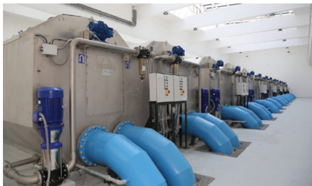
Each of the plant's 28 disk filter installations uses a Sulzer VMS pump (Image source: Metito)
