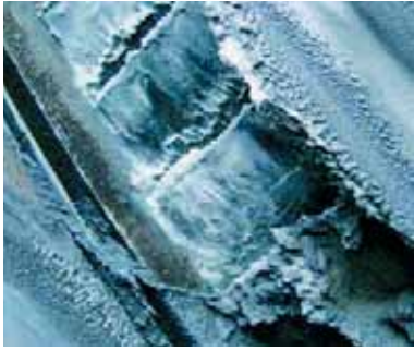
3 Hard scale deposit behind the turbine inlet nozzle.
