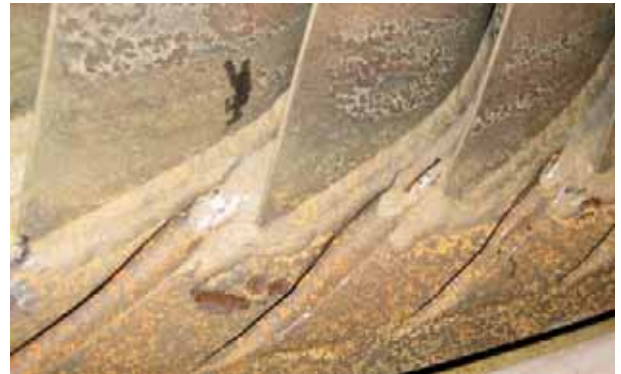
5 Erosion on the diaphragm caused by steam from the underground reservoir.
