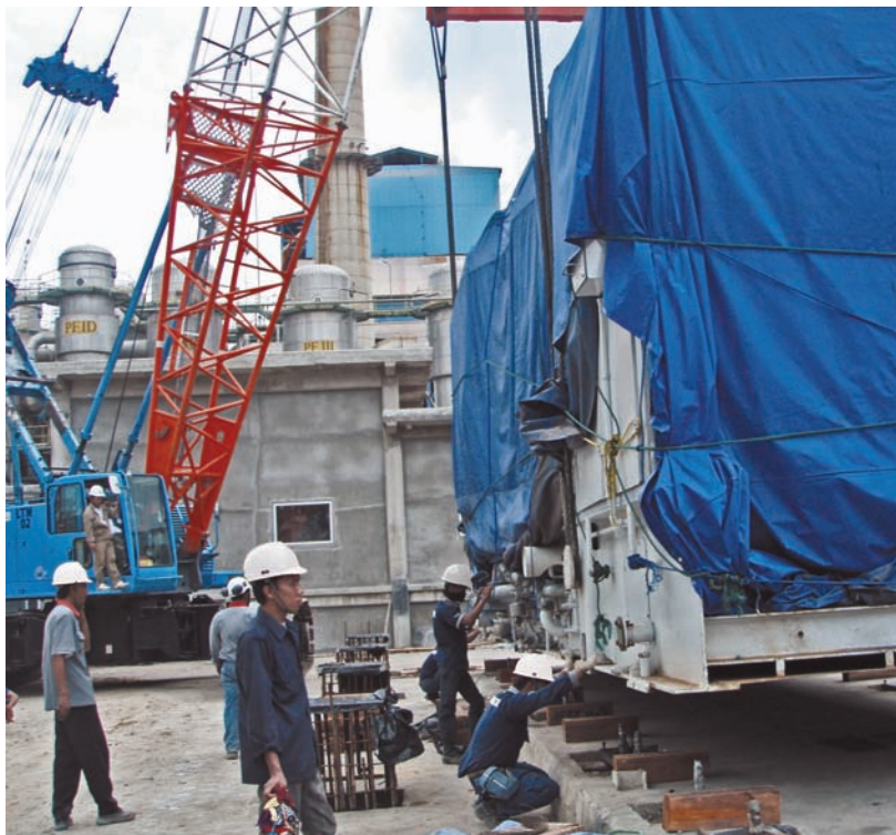
⑥ The gas turbine unit was directly loaded onto the foundation, and prealignment checks were continued.
