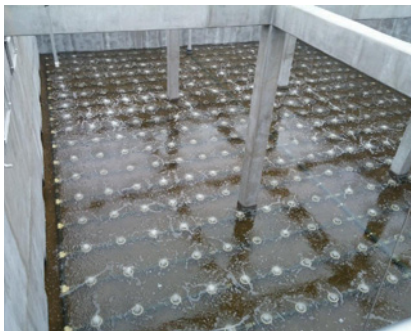
The old basin with new Nopon aeration system
