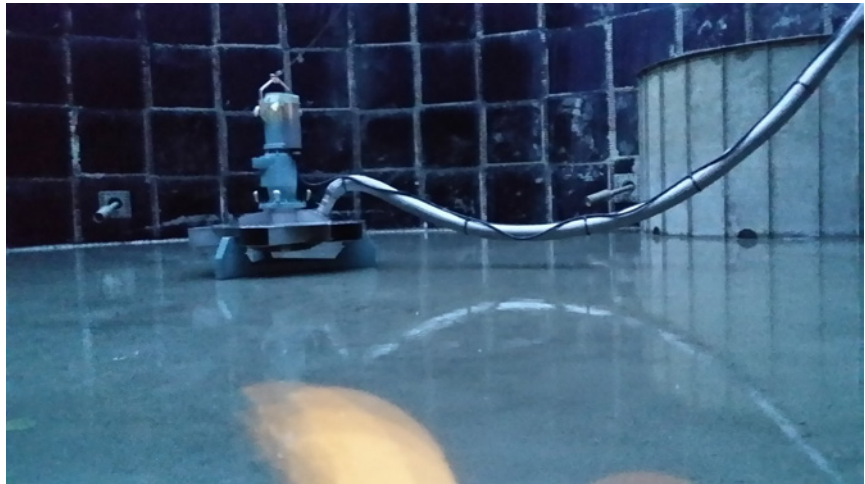
The OKI 2000 E-37AM with air hose at the bottom of a circular aeration tank.
