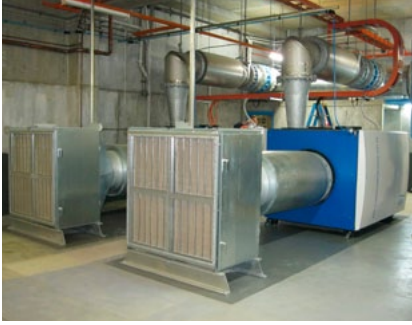
The Surbiton Park compressor room
