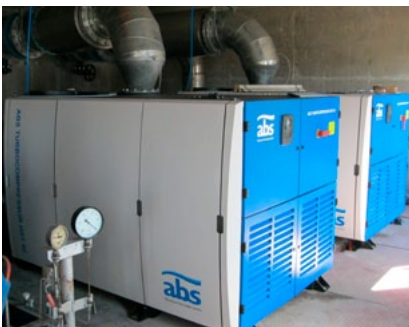
The Sunbury compressor room
