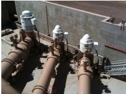
Vertical pumps at the 91st Avenue WWTP pump station
