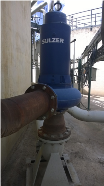
A dry-installed XFP 201G-CB2 PE110/6 pump for sludge recirculation
