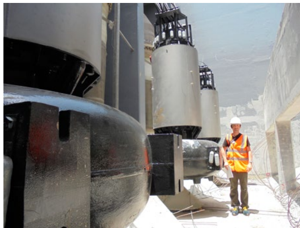
Gabriele Casella at the Al-Khumra pumping station
