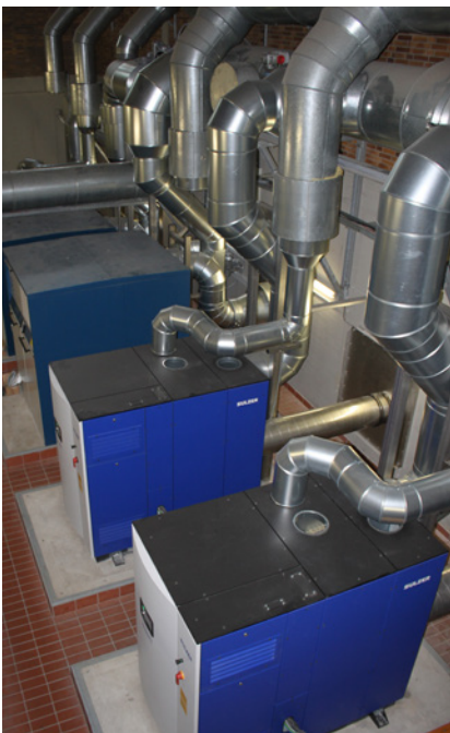
The new Sulzer HST 20 turbocompressors
