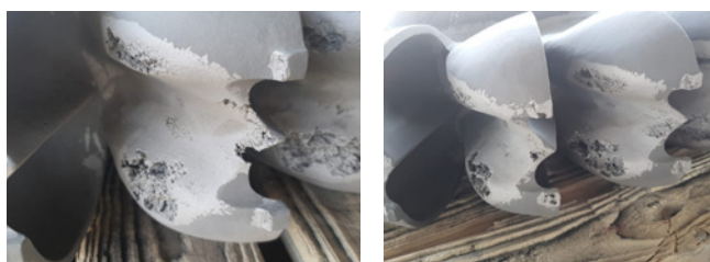
1. Wear and erosion visible across multiple buckets
