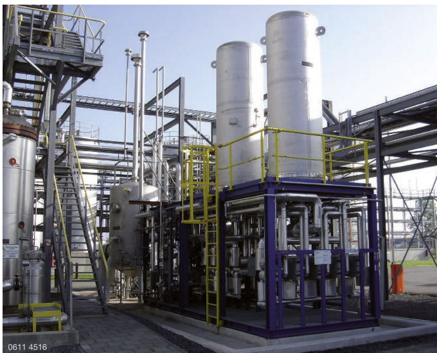
Skid mounted PERVAP™ membrane plant
