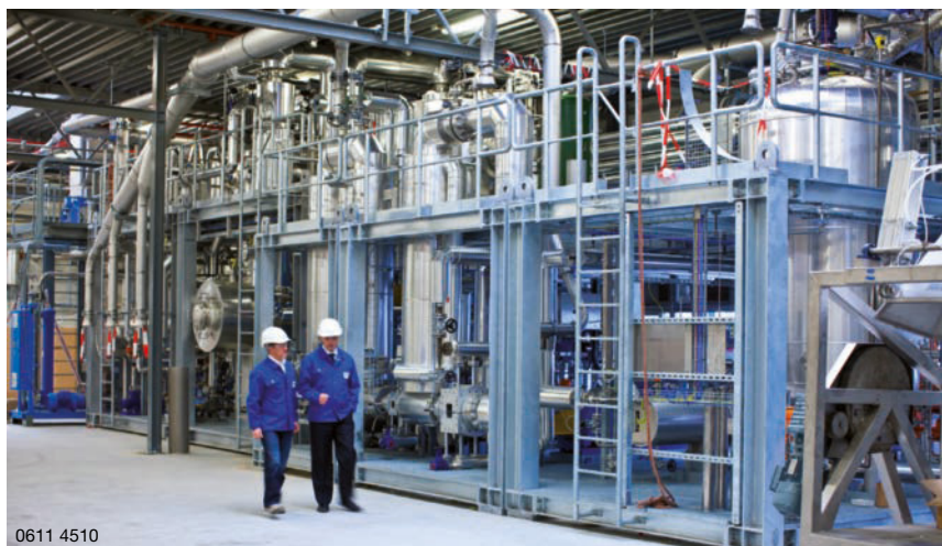
Skid mounted production unit for biodegradable polymer (PLA)
