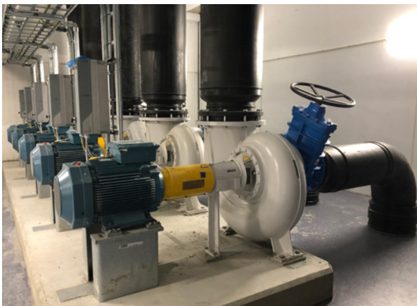
Five AHLSTAR A43-500 recirculation pumping units for brackish water
