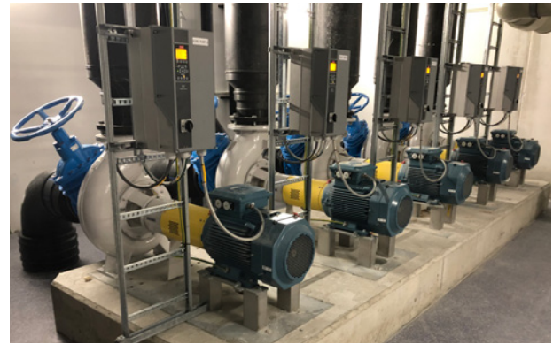
Five BE325-2532 recirculation pumping units for brackish water
