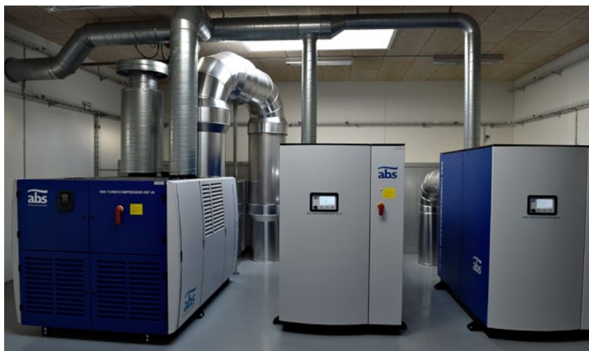
From the left: Turbocompressors type ABS HST40-350, HST20-6000 and HST20-4500
