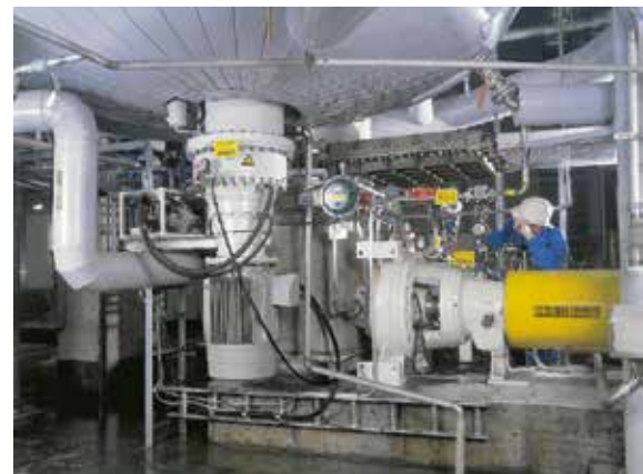
Fig. 17. MC tower discharge pumping system.
