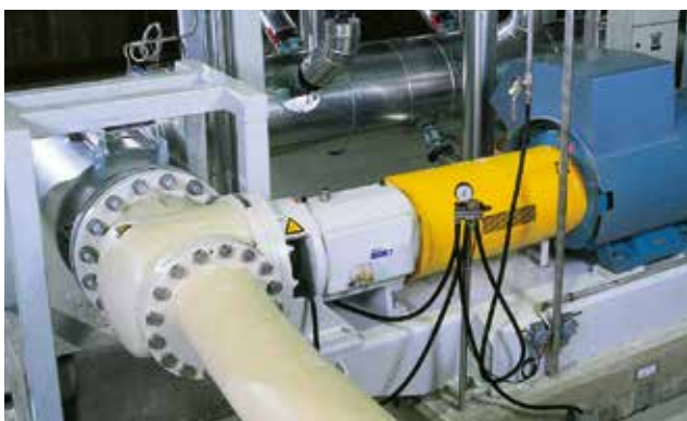
Fig. 2. MC equipment applications in a modern bleaching plant.
