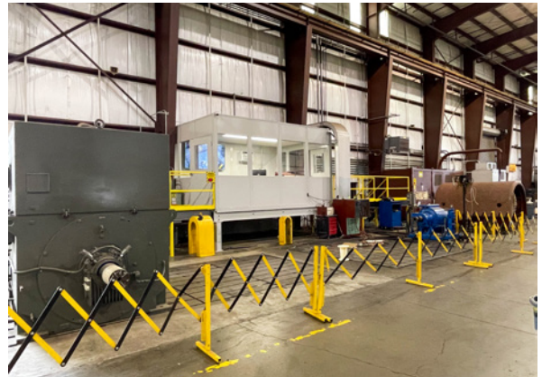
Multiple testing facilities from 460 volts to 13.8kv
