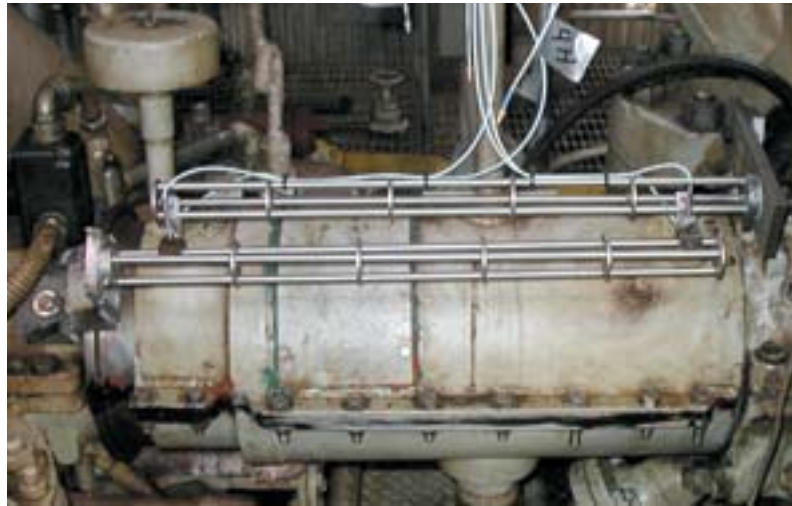
1 Alignment bars allow for an exact measurement of the centerlines of a machinery train. When the tolerances are met, coupling and bearing life are extended.
