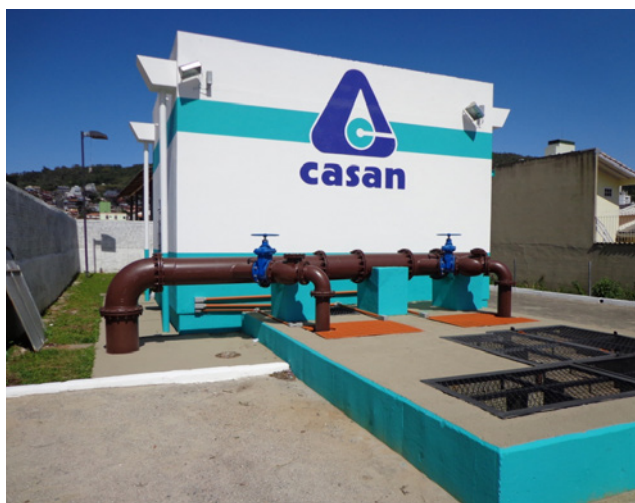
CASAN lifting station in Florianópolis: complete modernization with Sulzer equipment
