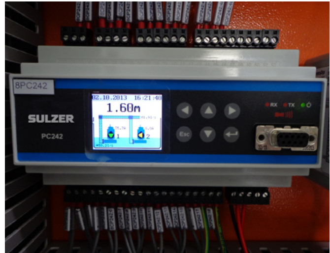
Pump controller type ABS PC 242 installed in CASAN lifting stations
