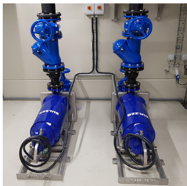
The XFP pumps working in a duty/standby arrangement, give the station a capacity of 25 liters per second.
