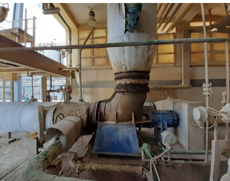
Evaporator circulation pump type CAHRM750K running at site (2020).
