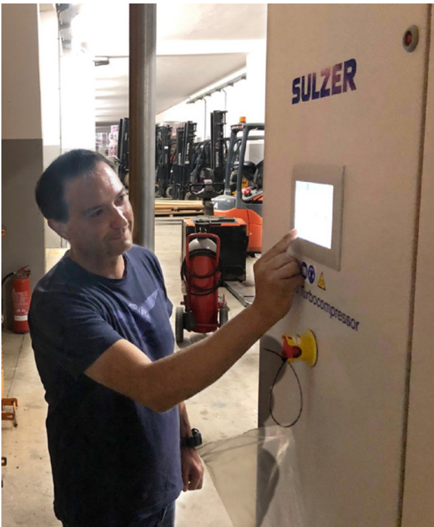
Mr. Buongiorno, Technical Manager of the converting line, setting up a new HSR compressor.
