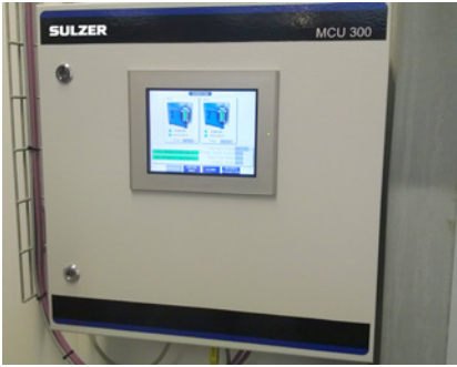
The master control unit in the compressor room
