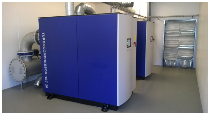
The two HST 20-6000-1-190s in the compressor room
