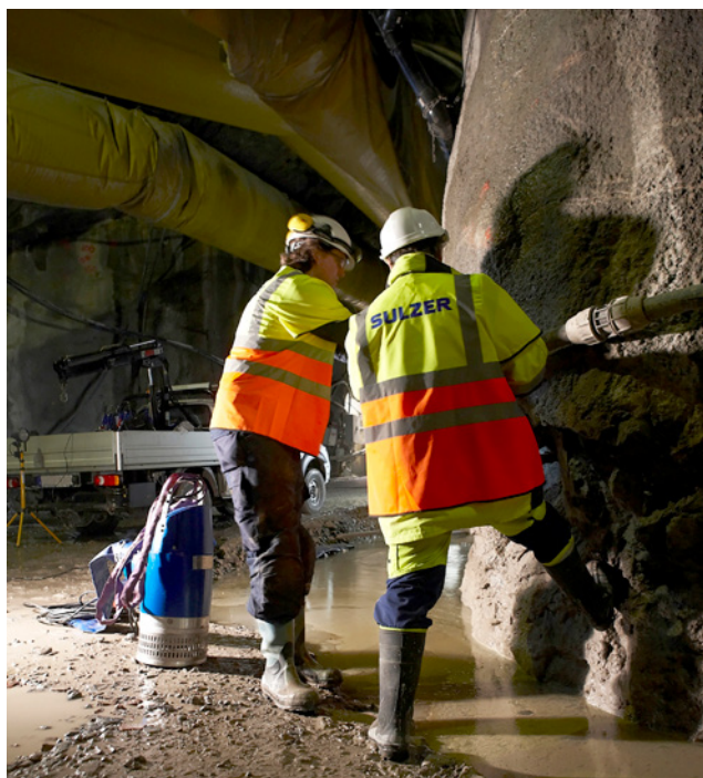
Dewatering installation with Sulzer XJ drainage pump.
