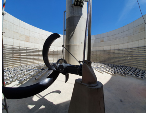
The annamox process uses 480 disc diffusers supplied by two HST 2500 turbocompressors
