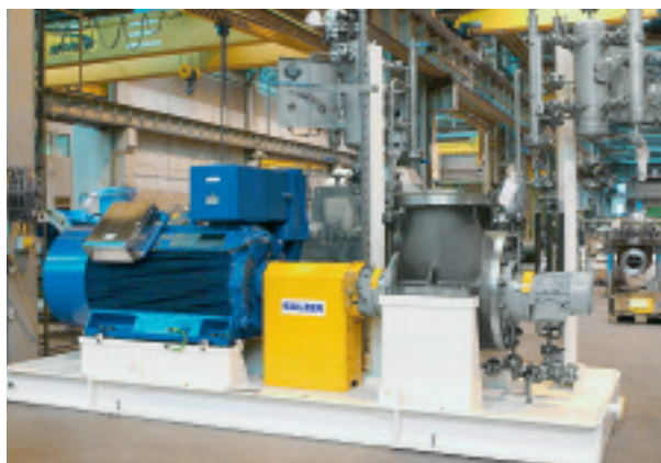
1 BBS pumps for heat transfer fluid circulation main.
