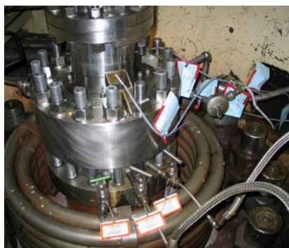
A Sulzer seal installed in a non-OEM reactor coolant pump
