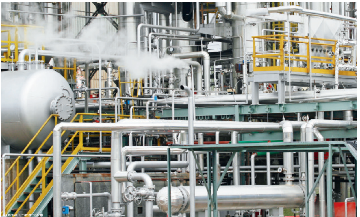
[1] Section of a refinery—the piping can be exposed to aggressive fluids under the insulation.
