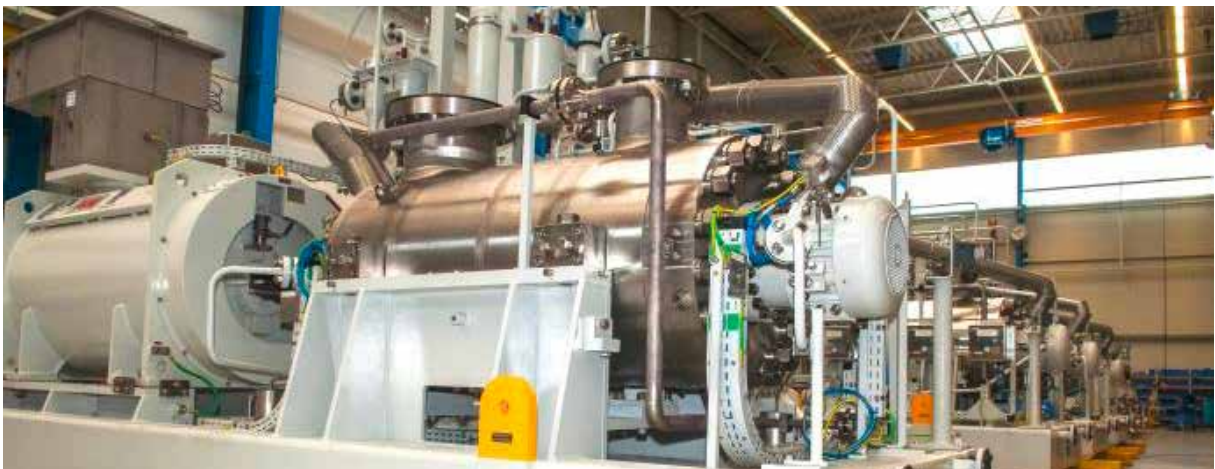
GSG cooling water pumps produced in Bruchsal.
