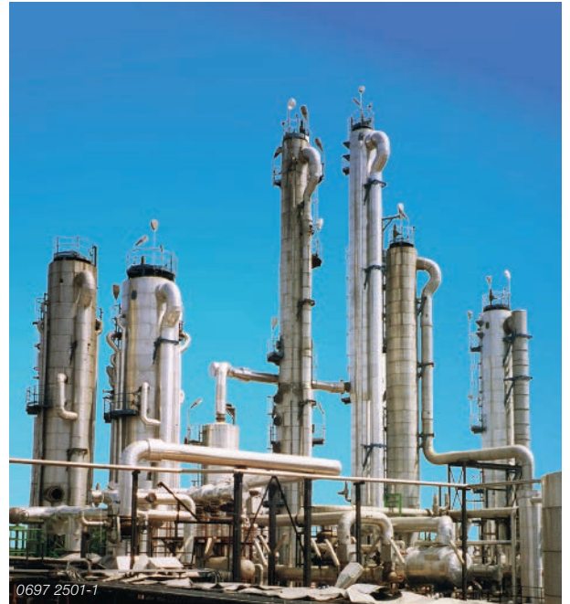
DMAc recovery plant
